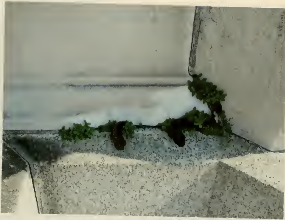
Figure 37: Material loss and invasive vegetation on pedestal
